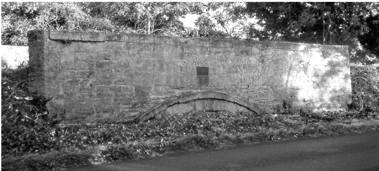
Fig. 1 The original A433 bridge over the Thames and Severn at Thames Head after the removal of undergrowth. The commemorative plaque above the arch reads :-
