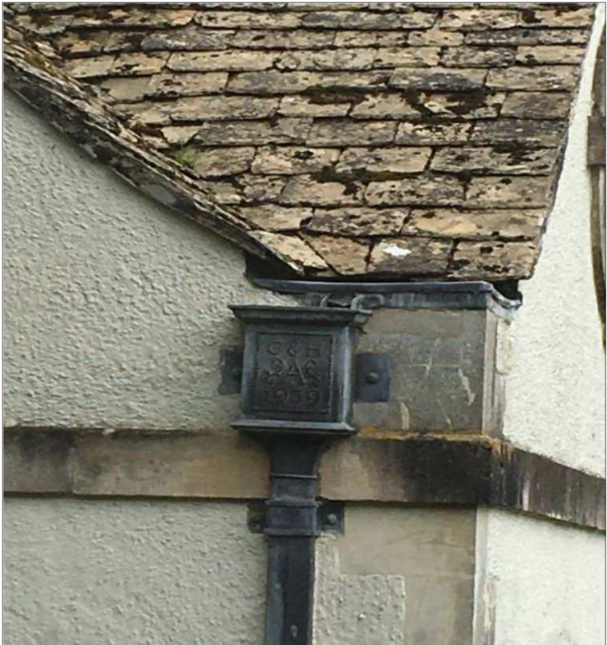
One of the lead rainwater hoppers produced for the 1939 rebuilt at Bodnant. It carries the inscription 'C&H' – a reference to Henry, Lord Aberconway, and his wife Christobel. Note the Cotswold stone tiles, as opposed to Welsh slates
