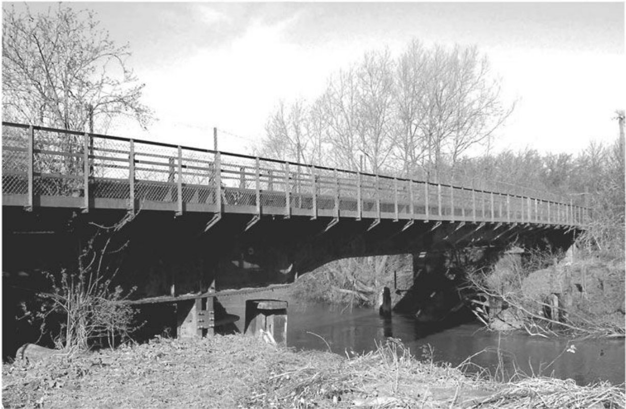
Llanthony Railway Bridge over the eastern arm of the River Sever in 2006. Hugh Conway-Jones
