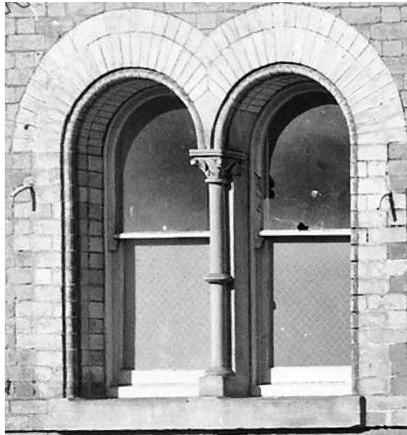
The sandstone windowsill and central mullion or colonette between the double round-headed windows on the South of the station
