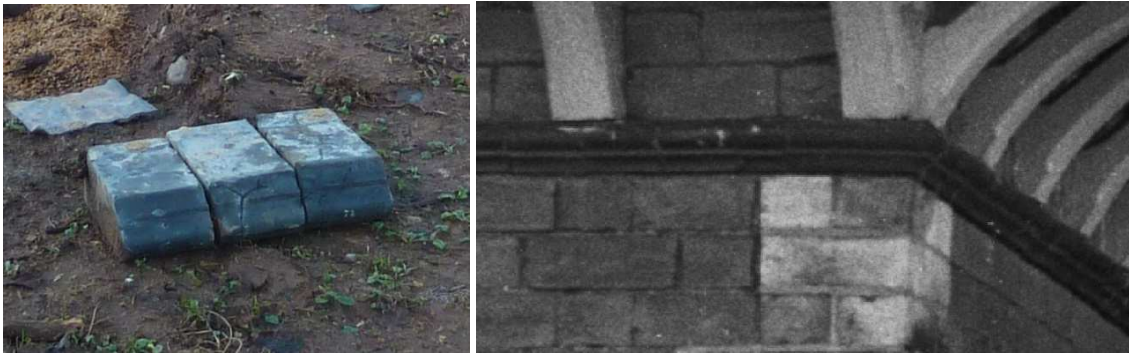
Some of the special blue string course bricks used at eaves level on the station in 1967
