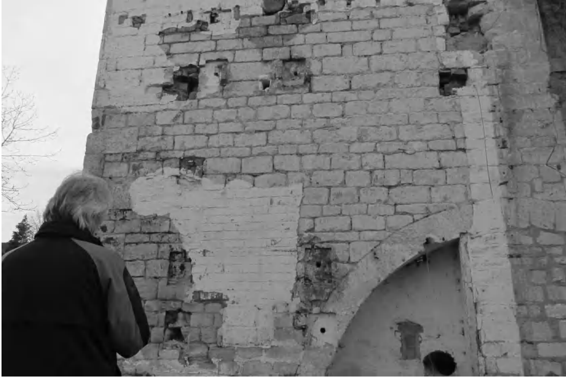
Figure 9 The main mill wall showing where the engine house once overlapped; the white line on the right indicates the one end wall. Note the earlier stone access arch, closed off when the engine house was added. Also note the openings cut high in the mill wall for the engine house roof beams and transverse engine supports, and the rectangular openings cut for reinforcement plates – these are thought to be associated with power transmission arrangements into the mill. The row of blocked upper holes carried the joists for the engine house’s upper floor.
