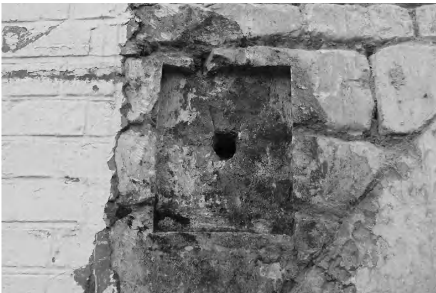
Figure 10. Close-up of one of the recesses cut for supporting plates. The bolt holes pass right through the mill’s wall. These presumably provided reinforcement for part of the power transmission arrangements.
